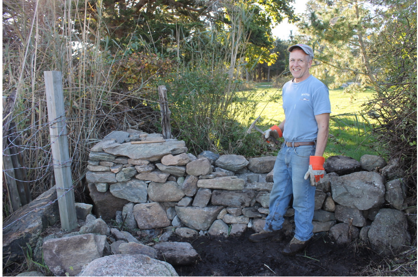
Chip Fales has spent many hours re-building a portion of the stonewall on the BBC western boundary line
