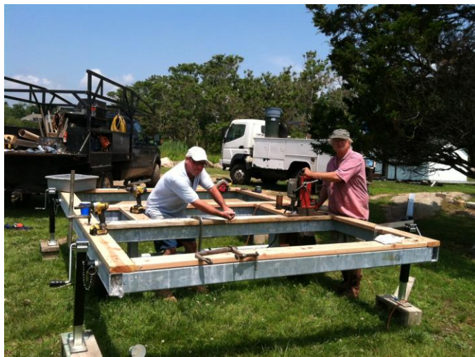
The "A Team," Eliot Benton and Mike Johnson, prepping the new galvanized steel trailer upon which they hoisted & mounted the Beach House.
